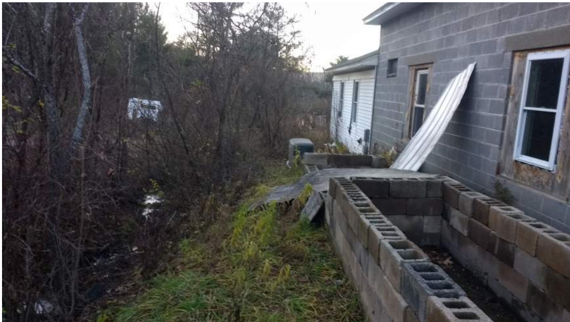
Rear of fire station – Brook can be seen on left side of picture.
